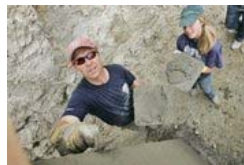
Melanie Issac held stucco for parent volunteer Rod Dubland this month as part of Vernon Christian School's construction project in a Tijuana neighborhood. (John Gibbins / Union-Tribune)
